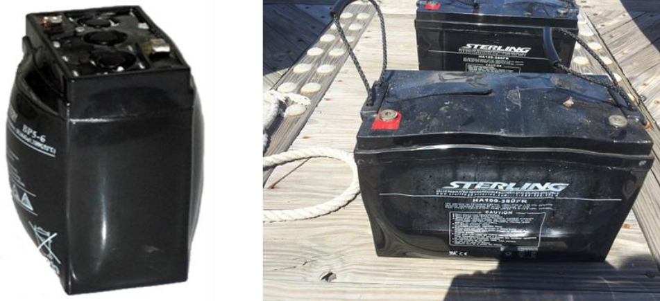
Figure 13: Swollen batteries due to excessive charging
