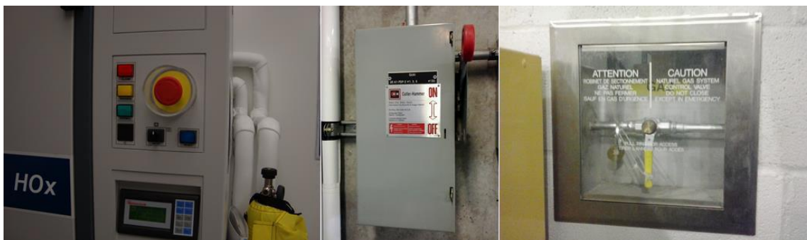
Figure 5.3.2-1: Examples of electrical and gas shut-offs
